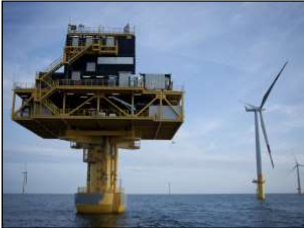
Converter substation offshore
