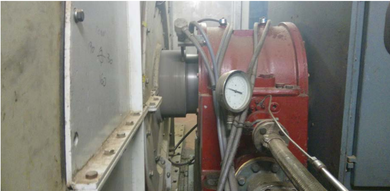
Figure 3. The shaft between turbine and generator.
